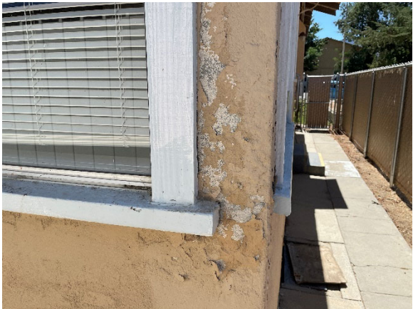
- Example of Exterior Deferred Maintenance-
