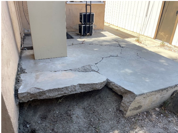
- Example of Exterior Deferred Maintenance-
