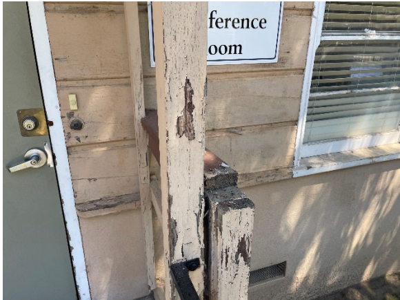
- Example of Exterior Deferred Maintenance-
