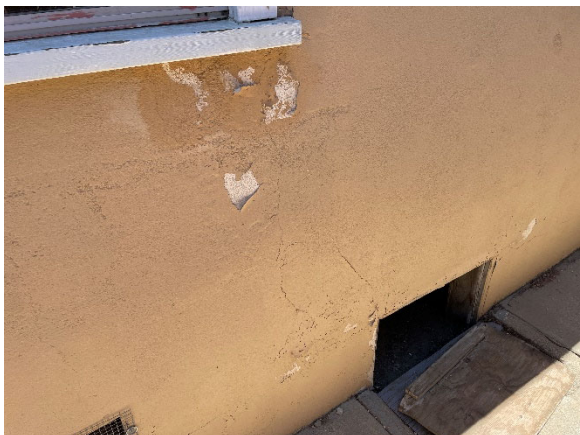
-Example of Exterior Deferred Maintenance-
