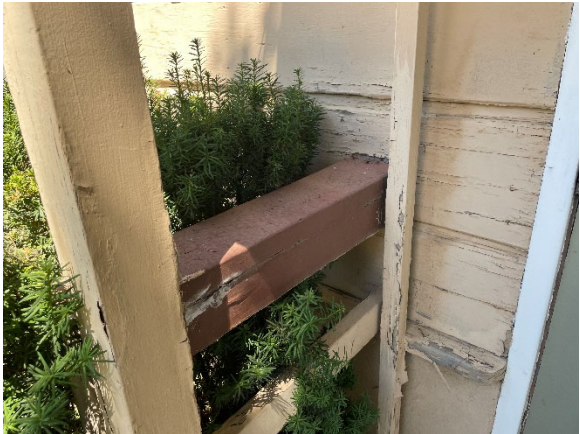
- Example of Exterior Deferred Maintenance-
